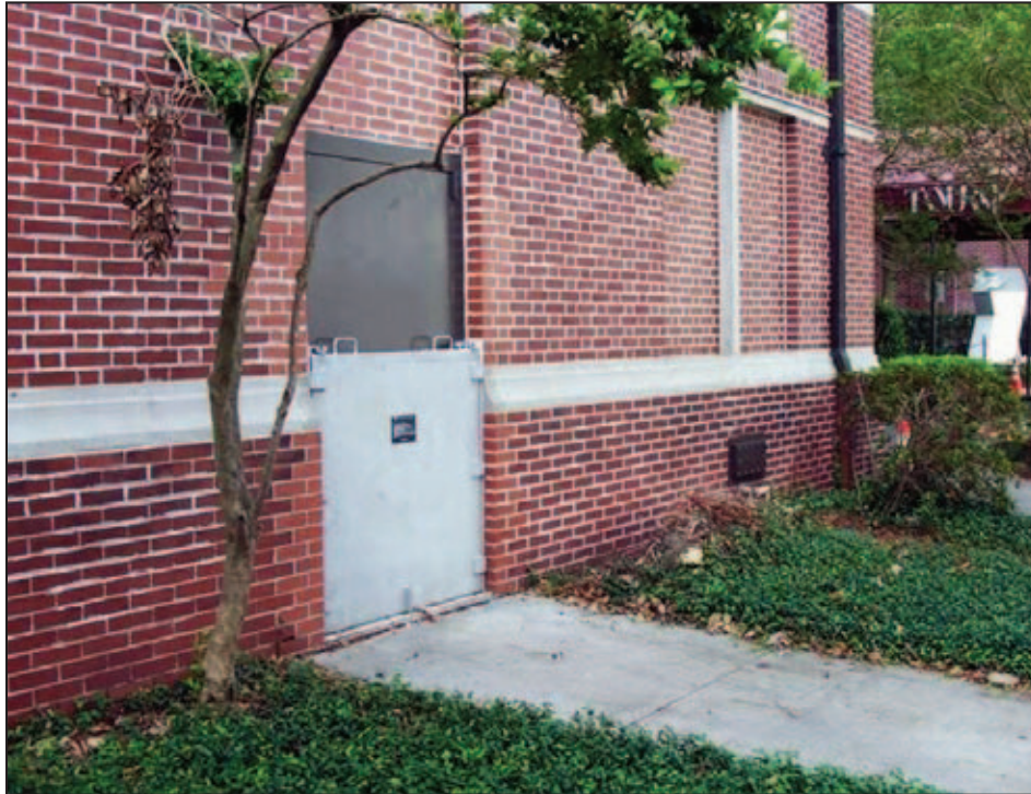
Figure 6-40. Example of a flood shield over a door
